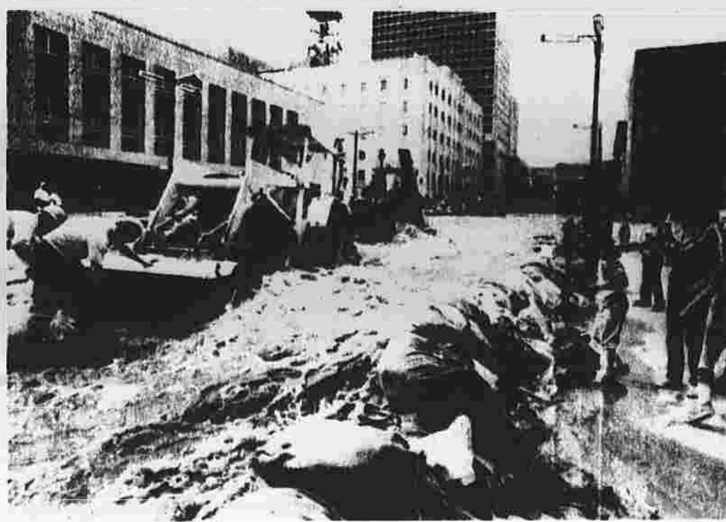
Flood control workers aided by heavy equipment look for manhole covers to pull Sunday in order to help direct the
