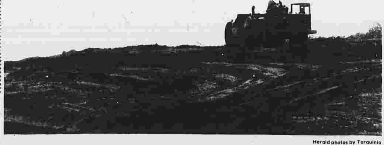
An earth mover levels a bluff on the east side of Buckland Street in preparation for a new highway bridge.
